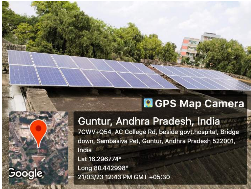
Solar Panel on College main building
